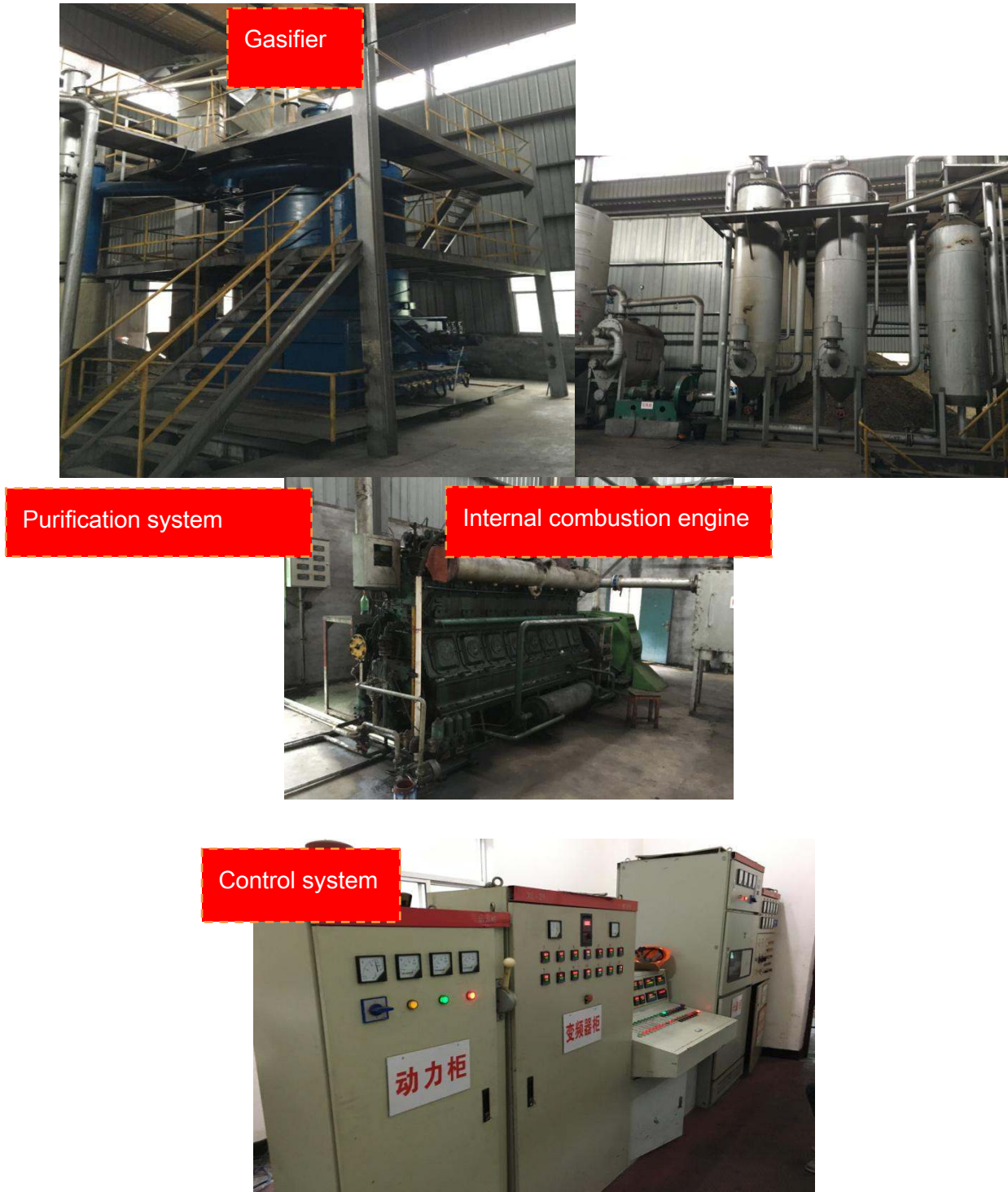
Fig.32 Bamboo gasification power generation system
